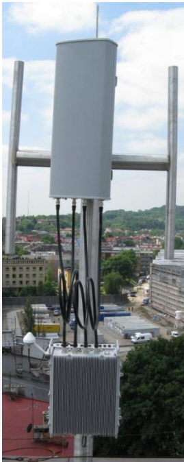
WiMAX Base Stations
